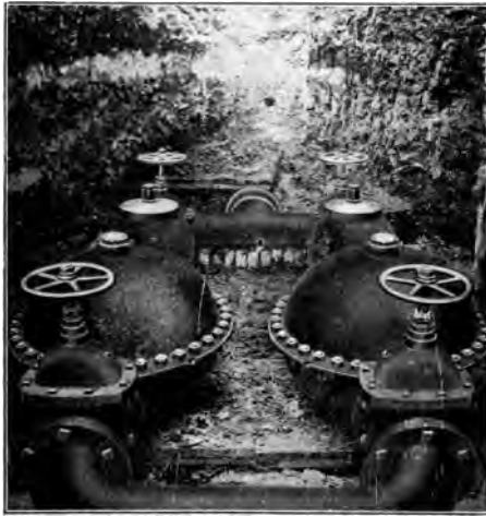
FIG. 324. — Battery of Water Meters.
